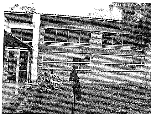
Looted and damaged building at the premises (Photo: RMA)
